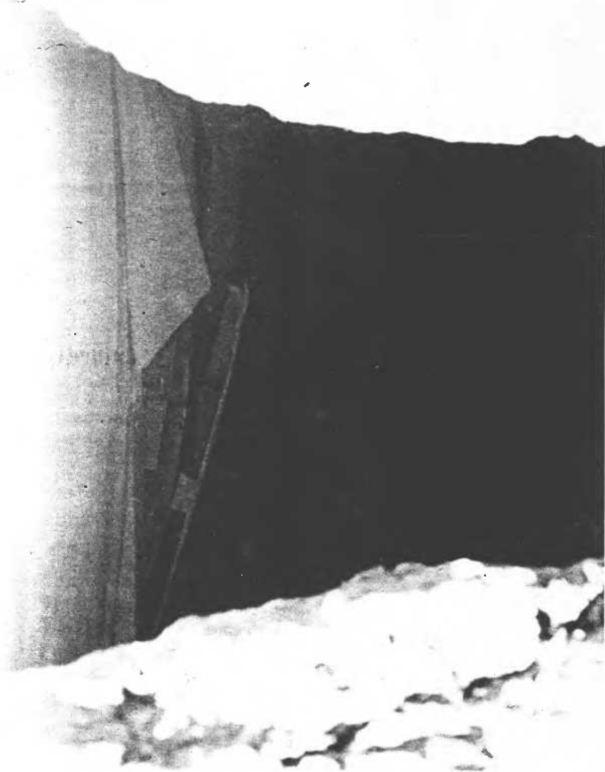
Fig. 3.6. Looking into the shelter after the rupture of the lower plywood-veneer sides of the doors. Since the veneer on the upper sides of the two partially broken doors and of two cracked doors remained intact, no earth fell into the shelter, and occupants would not have been injured by this unexpected type of failure of the most stressed of these very light hollow-core interior doors used for trench roofing.
