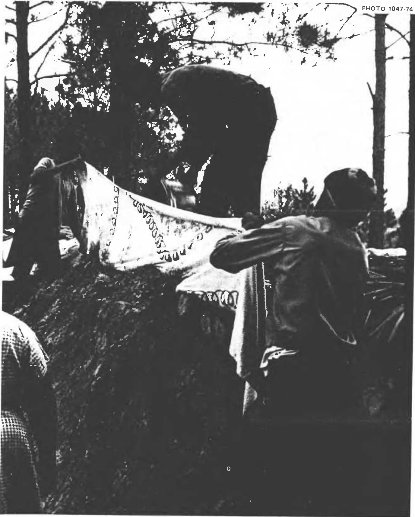
Fig. 5.22. Using an old bedspread to form an earth-filled roll along an upper edge of the essentially flat shelter roof of poles. The father is pouring earth out of a large bucket. These rolls made it possible to increase the stability of the earth covering around the edges of the roof, and also prevented heavy rains from washing any appreciable amount of shielding earth off the shelter roof.
