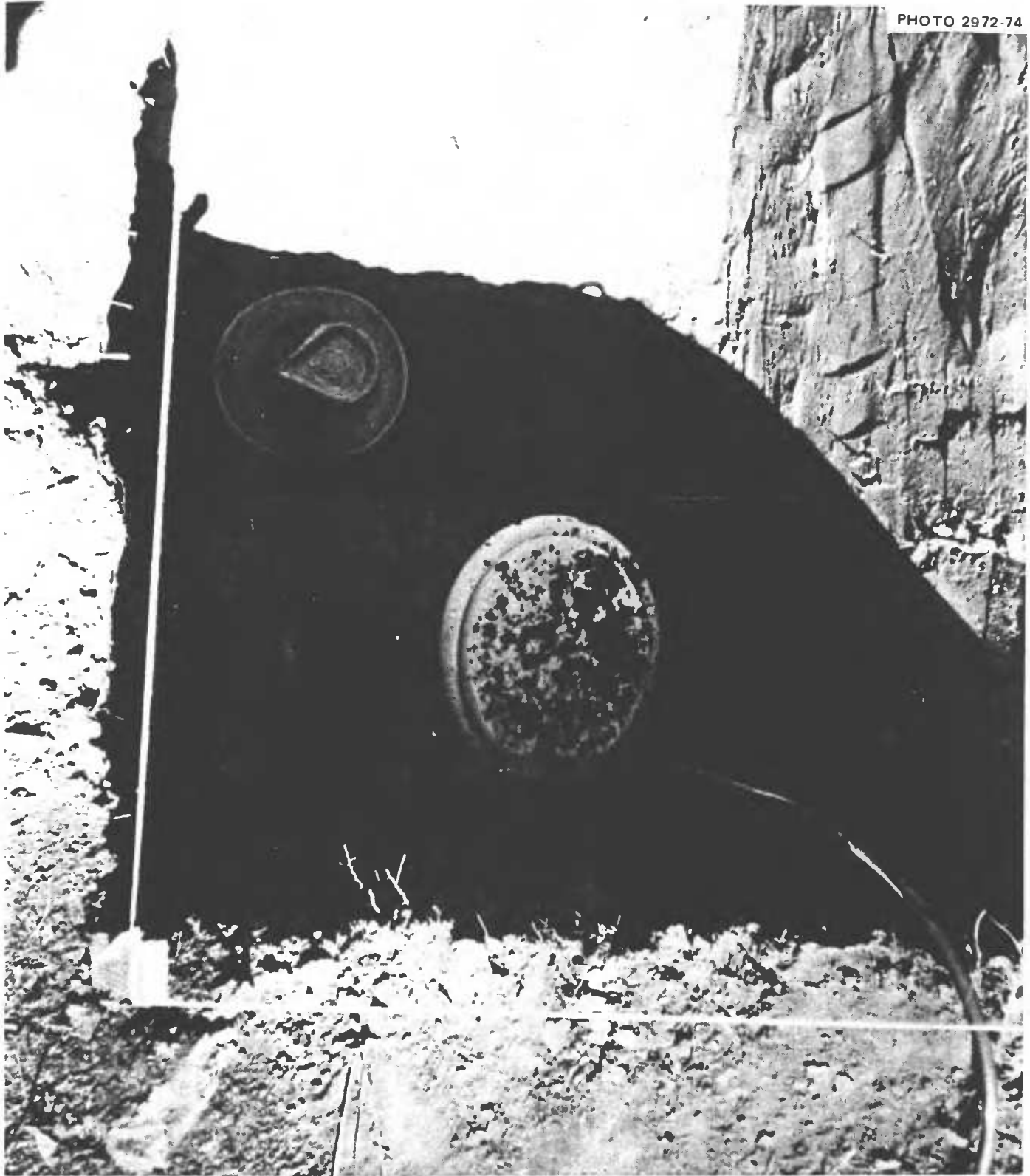
Fig. 4.29. View looking straight down on the installed toilet and its seat. The two assembled 5-gallon cans and the toilet bowl had been placed in a hole dug in the bottom of the shelter. A piece of \frac{1}{2} -in. plywood, in length equal to the 42-in. width of the shelter room and about 20 in. wide, served as the horizontal surface to which the toilet seat was attached. An appropriately sized, roughly elliptical hole had been cut in this plywood with a brace and bit and a cold chisel. The plywood base of the toilet was at floor level. Note the vent hose.
