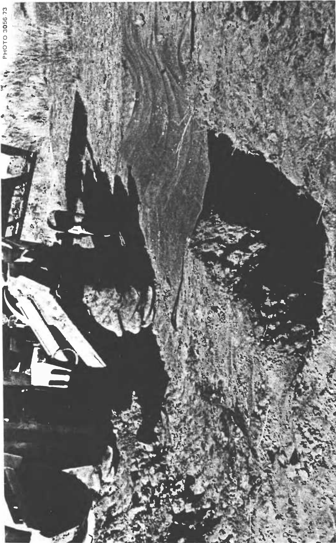
Fig. 3.12. Compacting the earth over one edge of the tarp. This edge has been placed in one of the two 16-in.-wide by 12-in.-deep rectangular trenches, each of which was dug parallel to and 3 ft from the vertical walls of the shelter trench. Packing with this wide-wheeled backhoe did not compact the earth as well as hand-tamping it with a pole.
