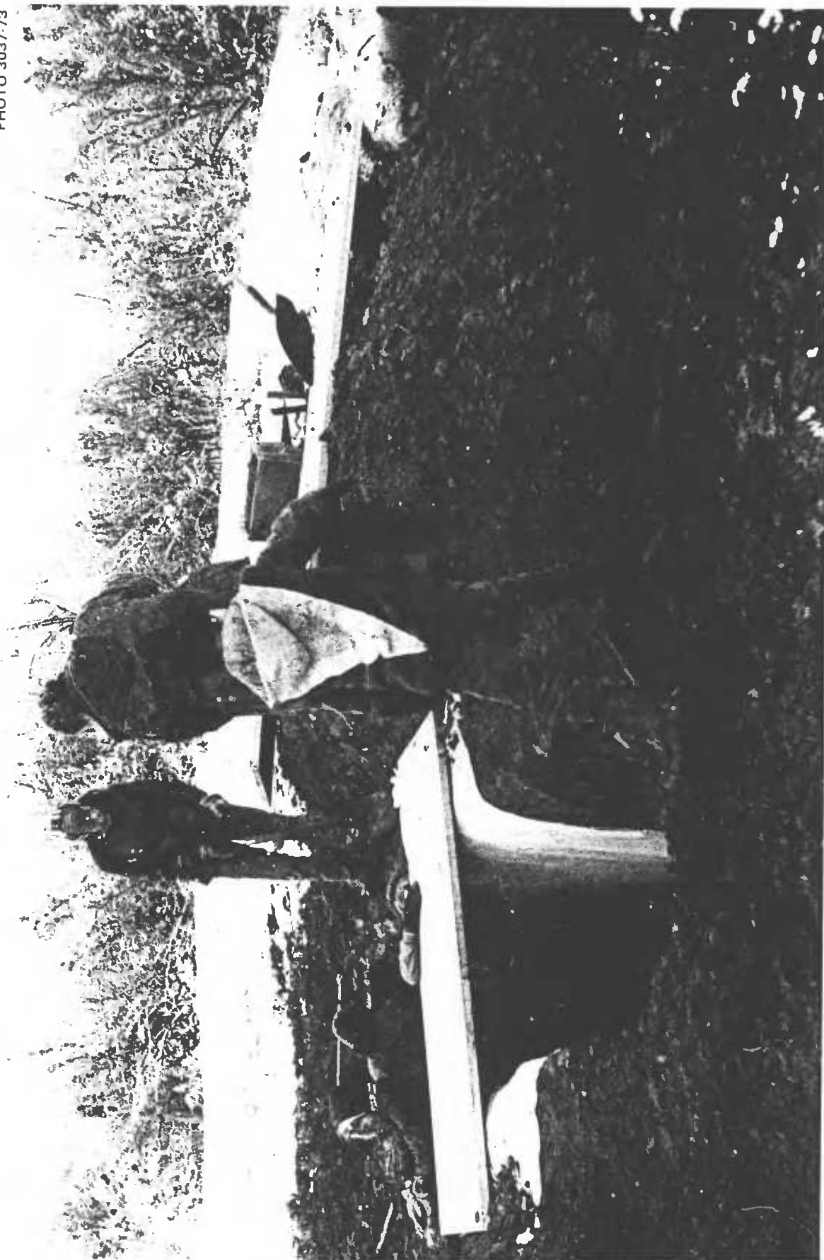
Fig. 2.9. Placing the first of six interior, hollow-core doors over the completed trench. The earth on the wall-lining sheet was removed before the second door was positioned.
