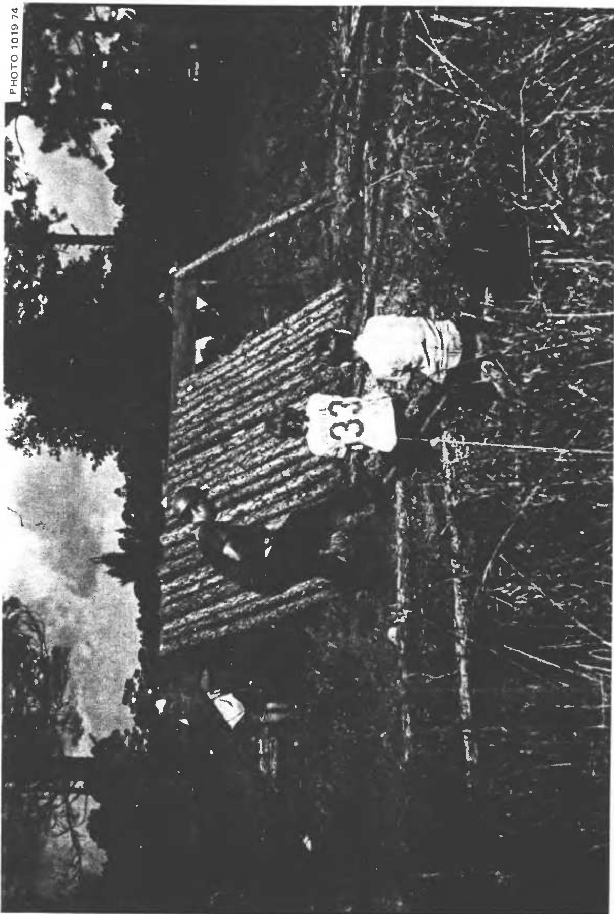
Fig. 5.45. Chain saw operator using a templet to cut an upper end of a wall pole at the specified 54^\circ angle and 9-ft length on its short side. The templet was made from a wide 10-ft board, with one end cut at 54^\circ . A nail was driven 9 ft from the end of this 54^\circ angle; the squared-off base of the pole was placed against this nail.
