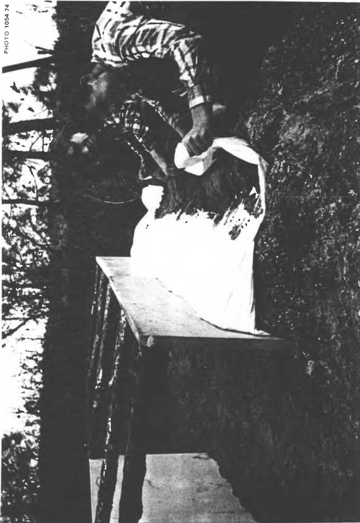
Fig. 5.58. Workmen building the first prototype of a shelter with vertical interior walls consisting of 2 or 3 rolls, stacked one on top of the other. This photo shows the workers forming an earth-filled "hook," which holds the part of a sheet forming the upper side of a roll in place, so that especially the vertical inner side of the roll will remain in place when the door form is removed.
