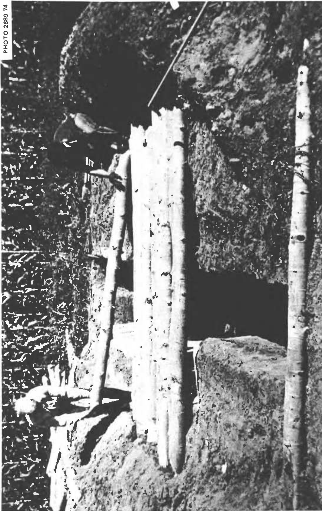
Fig. 4.7. Placing the 9-ft roof logs, all 2 ft off center, over the 3\frac{1}{2} -ft-wide main trench. A shelter in firm earth such as this, with 9-ft roofing logs positioned 2 ft off center, would enable the builders to widen their shelter to a 5\frac{1}{2} - or 6-ft width and to deepen it to standing height. If their home and community were destroyed, the family could live in such a rainproof dugout for months, if necessary, while minimizing their radiation doses and being more comfortable, in cold weather, than if living in a tent or shack.
