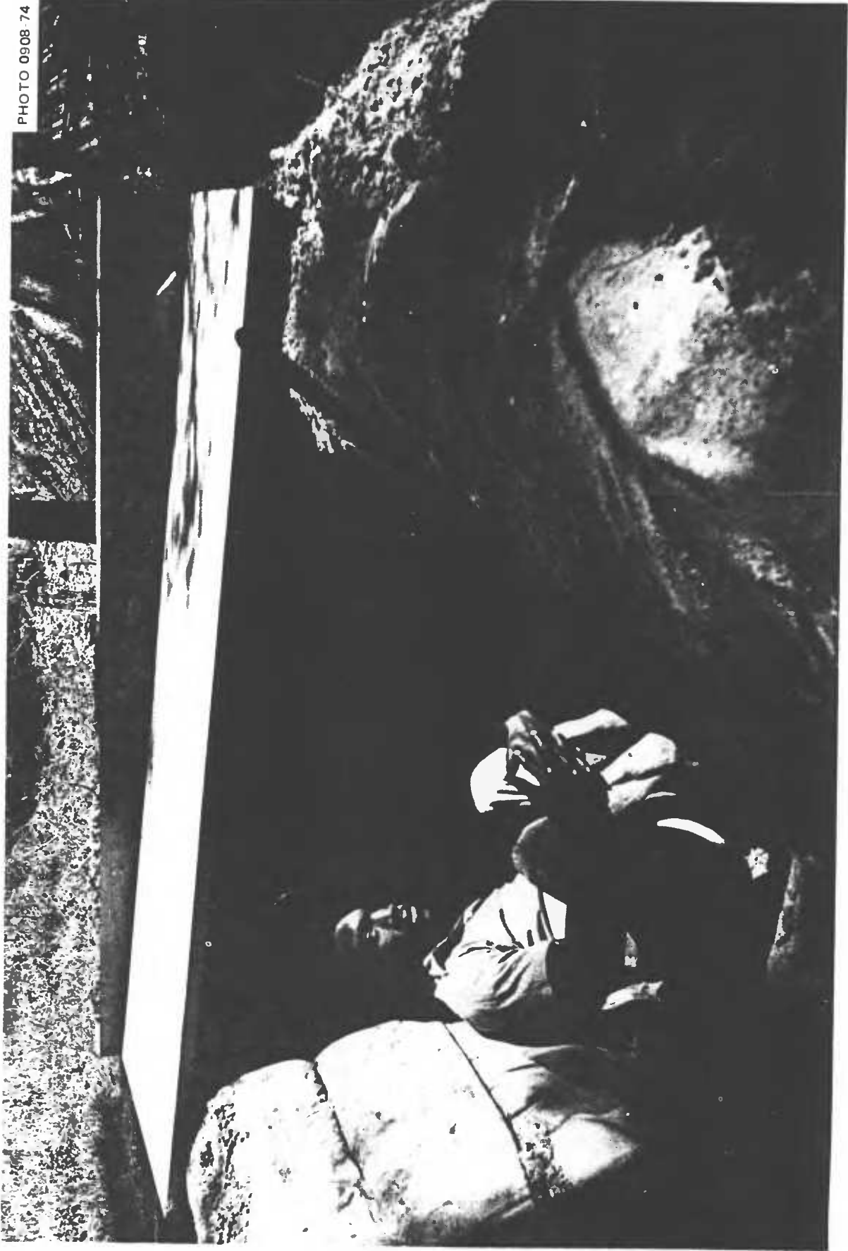
Fig. 5.55. The first of the hollow-core doors used to roof the initial prototype of an above-ground, door-covered shelter using earth-filled rolls for its walls. Since at this time Kearny did not realize that earth-filled rolls made of bed sheets or 4-mil plastic film could be used to form strong and stable vertical walls, these rolls were made sloping inward. This resulted in the free span of the roofing doors being about 5 ft wide. When the single-thickness doors of this roof were loaded with 15 in. of heavy, sandy soil, they broke within 1 to 3 days, although the earth was dry and no rain fell. Humidity, however, was high.
