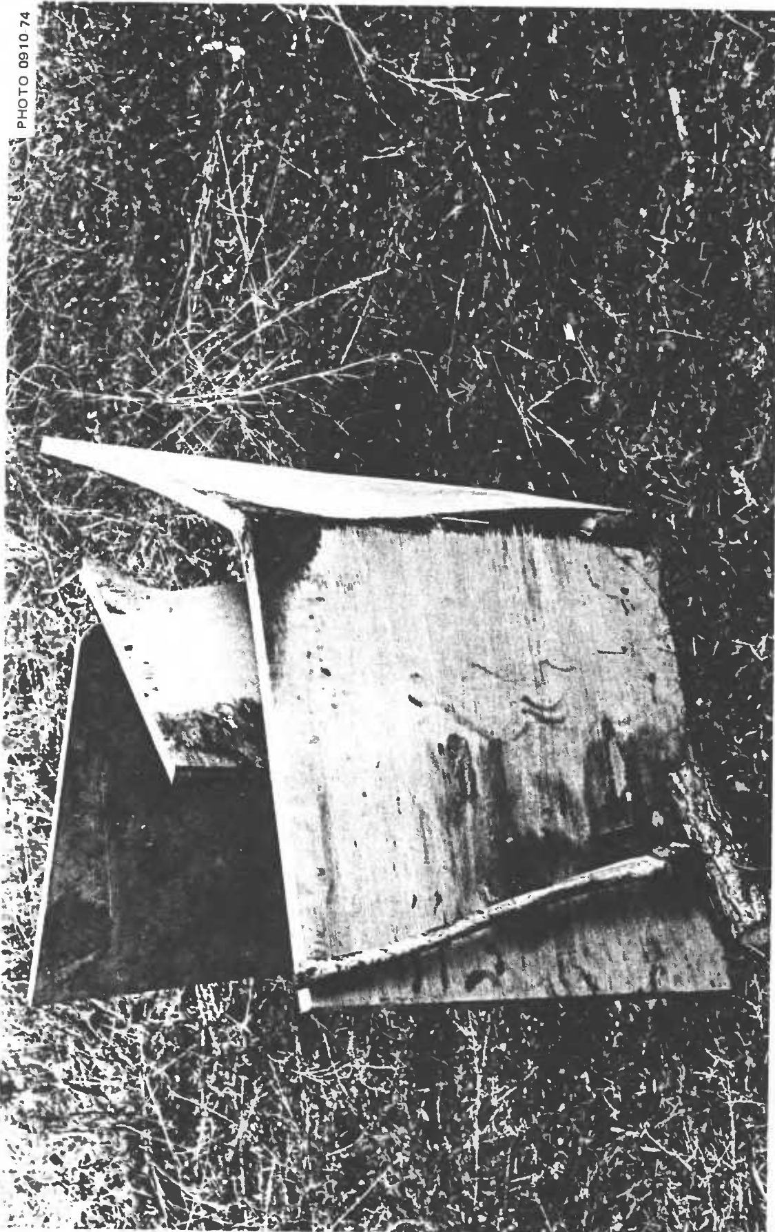
Fig. 5.56. Two of the broken roof doors after they were moved from the previously described shelter. Because the ratio of the depth of earth cover over these doors to the width of free span was too small, the centers of these broken doors fell to the floor of the shelter.
