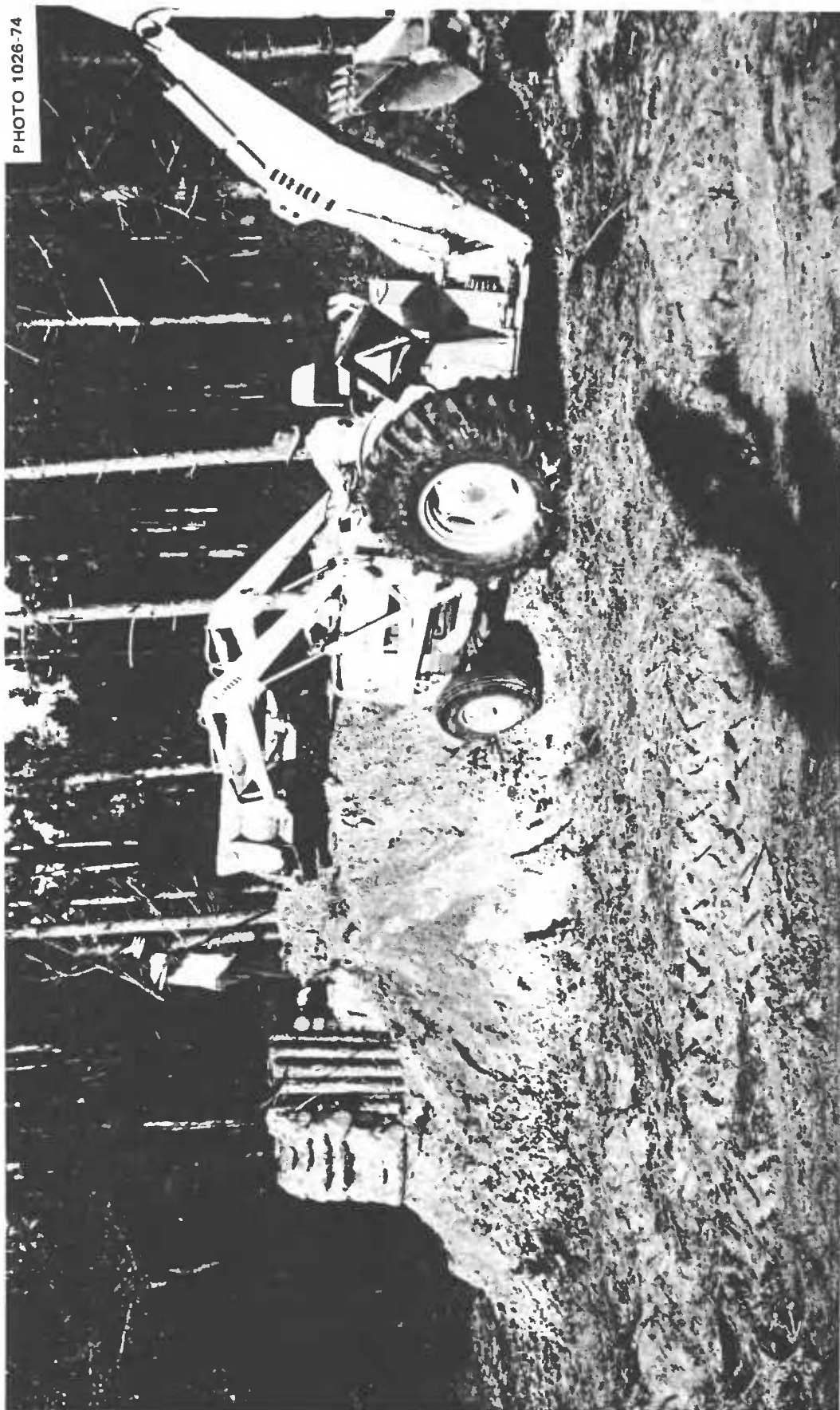
Fig. 5.68. Backhoe covering the unsuccessfully modified Small-Pole Shelter with three rooms built entirely above ground. The backhoe worked for almost 5 hours to place earth on this shelter to a minimum depth of 2 ft, because it could excavate only a little over a foot deep without getting stuck. The backhoe repeatedly had to lift itself out of the mud on both its buckets, although this work was done toward the end of a long dry spell.
