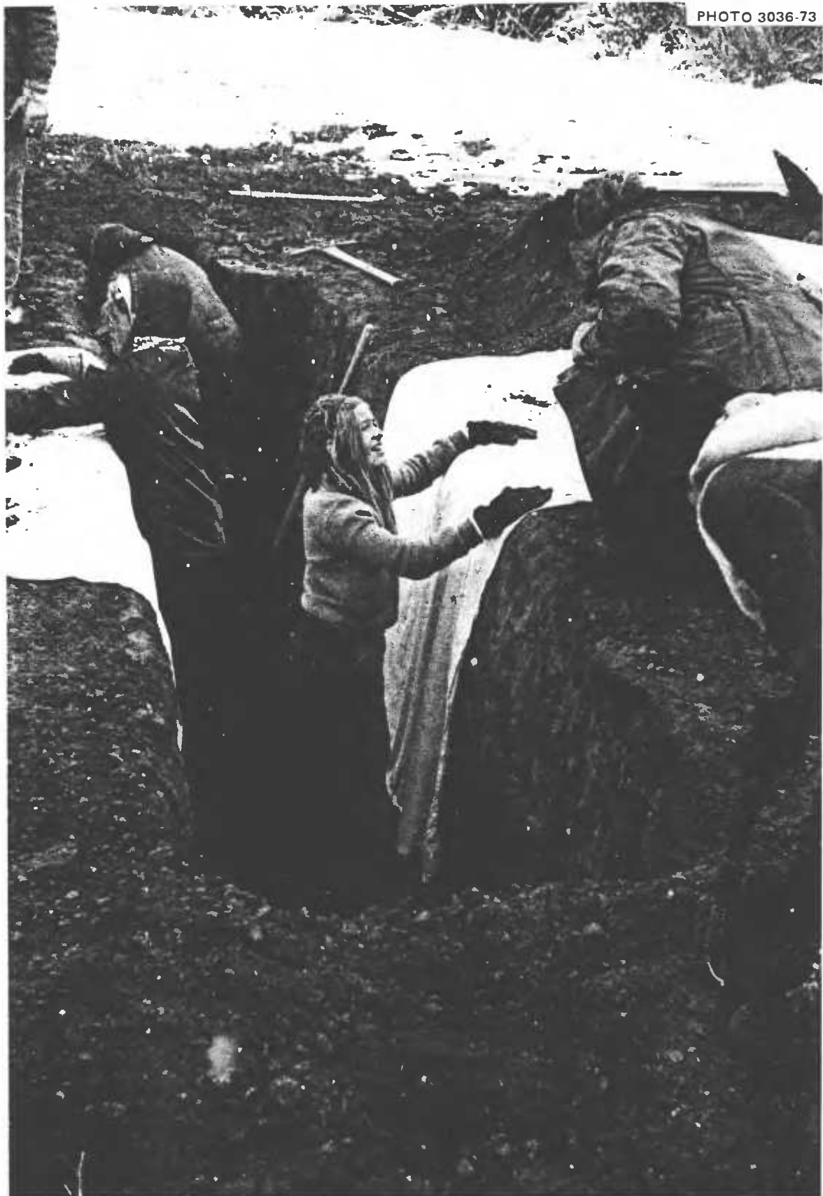
Fig. 2.8. Placing bedsheet coverings on the 4\frac{1}{2} -ft-high trench walls. Such coverings make the trench cleaner, warmer, and easier to illuminate.
