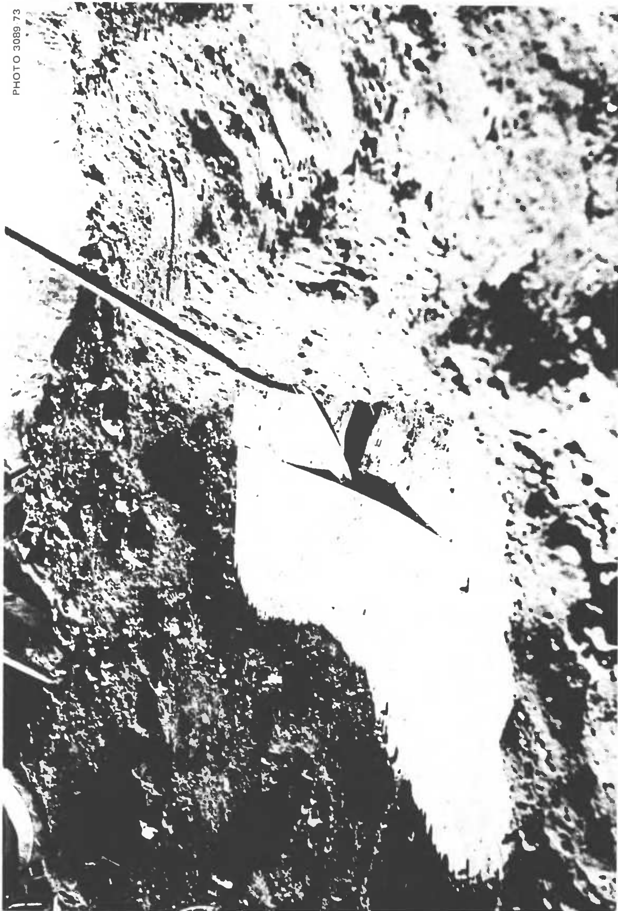
Fig. 3.8. Another view of the most downward-bowed upper veneer of a door. The ratio of earth cover to free span was 2\frac{1}{2}:40 , that is, greater than \frac{1}{2} . A ratio of \frac{1}{2} , or greater, is usually required for the development of effective earth arching in the earth cover over a beam capable of being bowed downward sufficiently without breaking by the weight of the earth and/or downward pressures applied to the surface of the earth cover.
