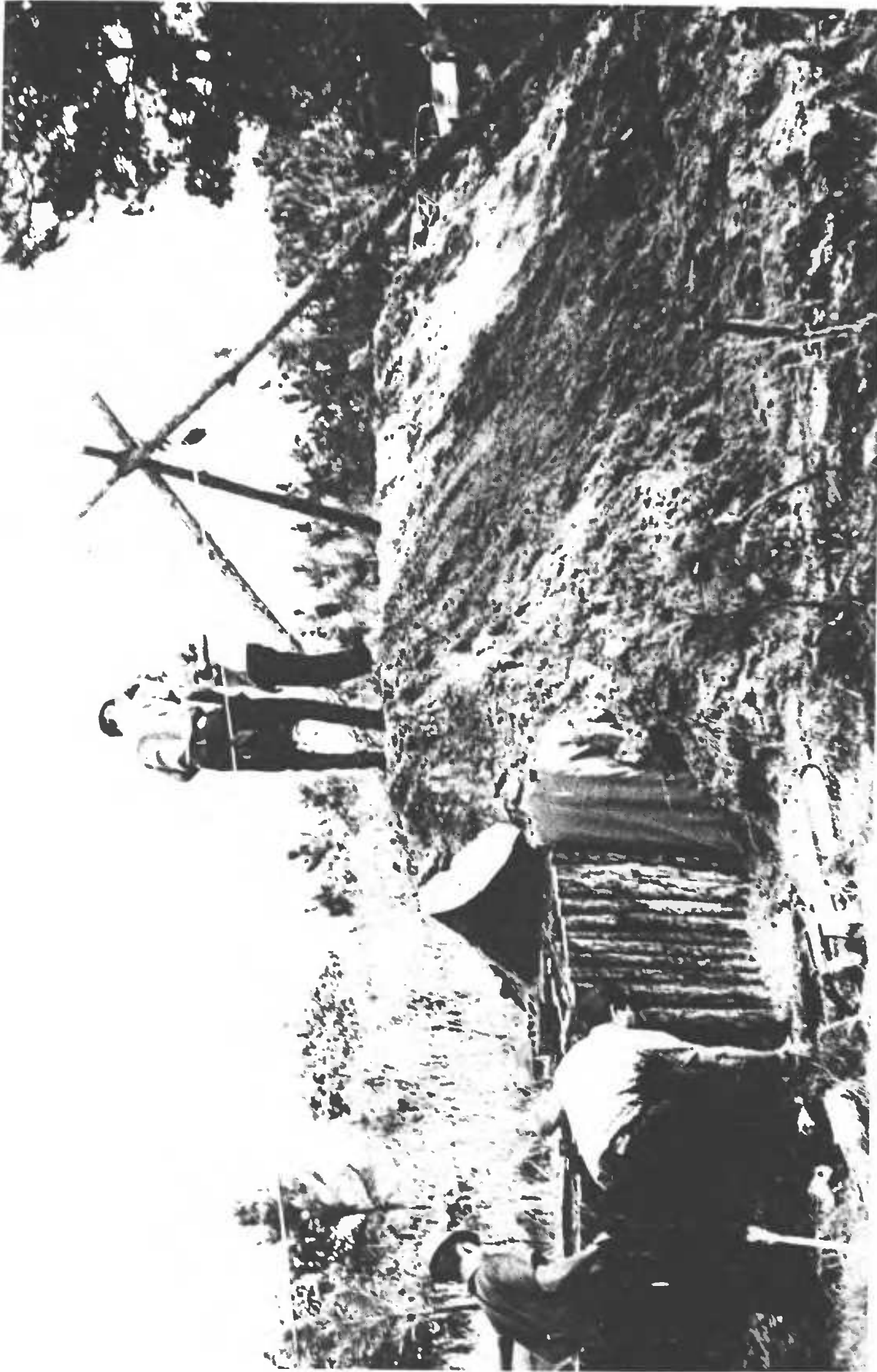
Fig. 5.51. The pulley conveyor system actually wasted energy and time, since earth had to be lifted in a 5-gallon paint can up to the hook on the movable pulley; then the earth-filled can was pushed up the upward-sloping nylon rope to a position several feet above the top of the shelter. Then most of the earth rolled down below the top of the shelter, obviously wasting thousands of foot-pounds of work.
