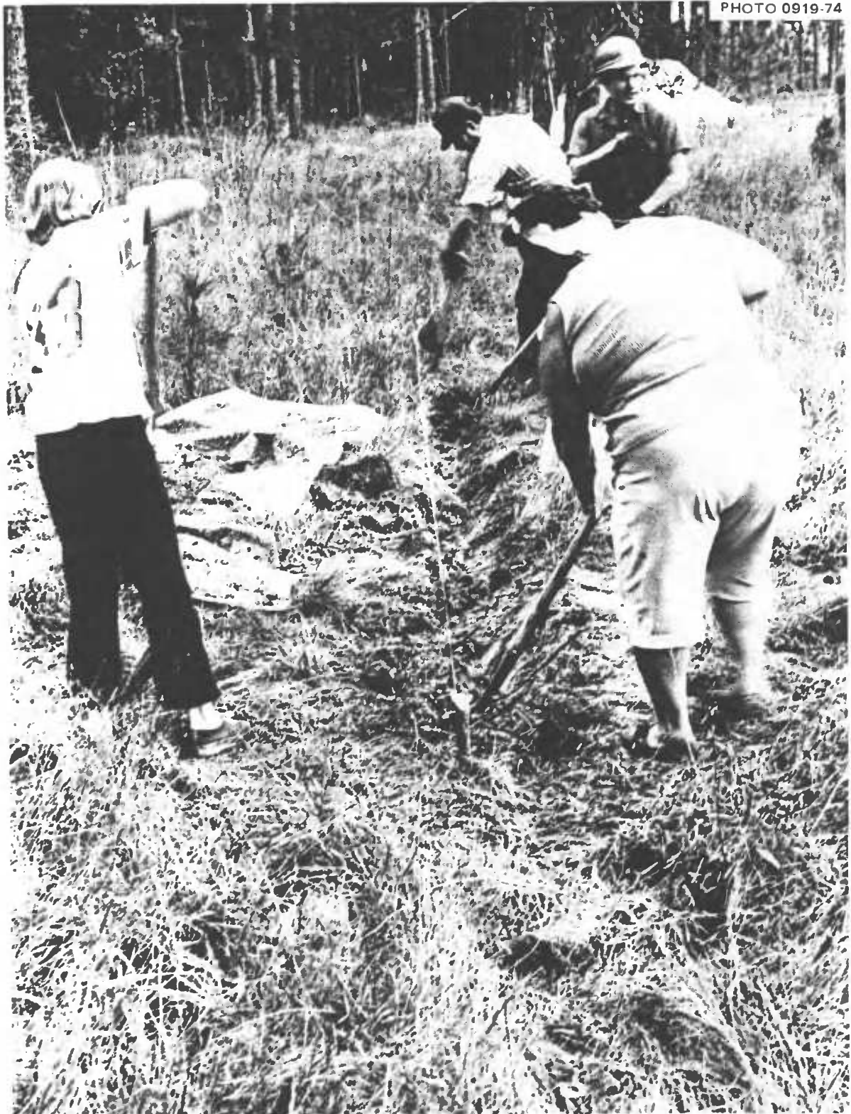
Fig. 5.42. Starting to build a 21-person above-ground A-Frame Pole Shelter. Five families, having 22 persons in all (including two babies and three adults unable to do heavy work) built this shelter with a main room 21 ft by 13 ft wide. The roof poles (not shown) had a minimum small-end diameter of 3\frac{1}{2} in. and sloped approximately 36^\circ . This photograph shows one of the 6-in.-deep, "V"-shaped trenches being dug to secure the lower ends of the 9-ft roof poles, that measured 9 ft on their short sides.
