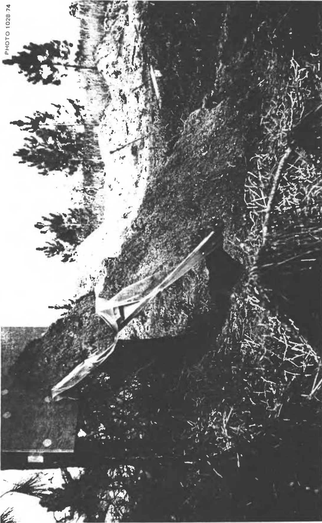
Fig. 5.64. The door was loaded with about half the specified average thickness and weight of earth, due to earth falling off the sides.
