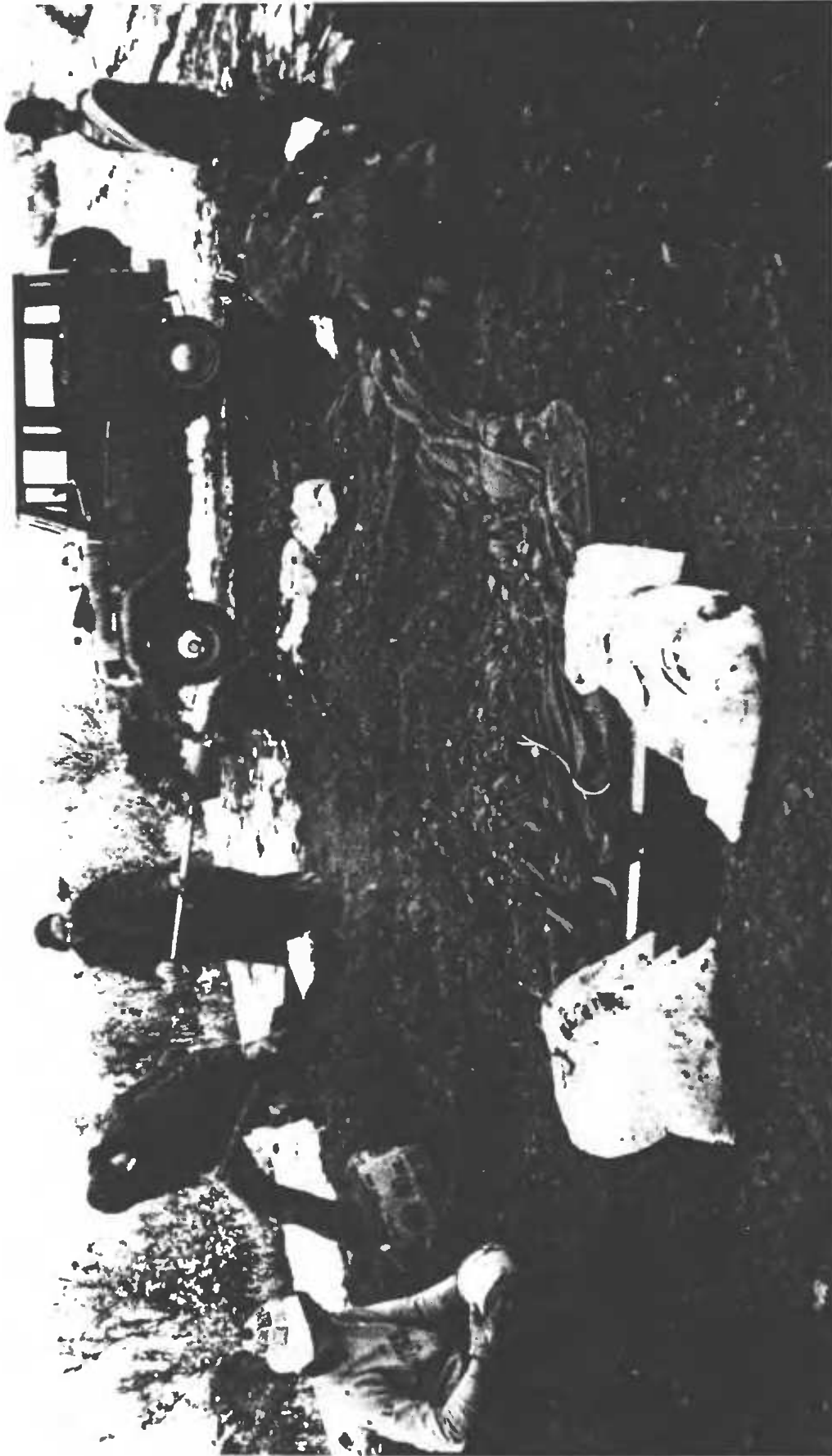
Fig. 2.10. Covering the water-shedding "buried roof." This family used a tent, due to a desire to save their shower curtains and most of their plastic table cloths, etc.
