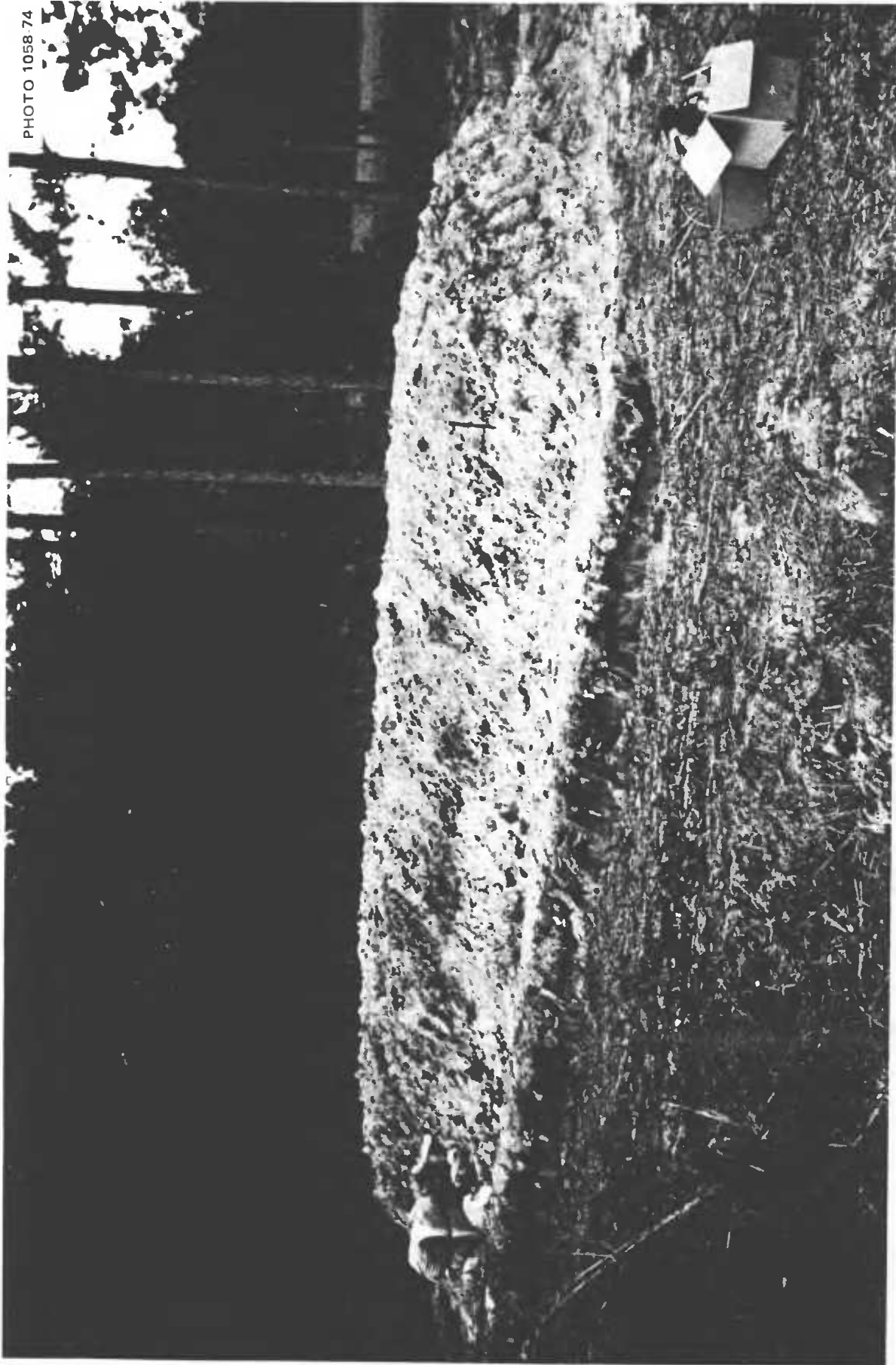
Fig. 5.9. The completed shelter, after a full 15 in. of heavy, wet, sandy earth had been piled on top of the roofing doors. These doors had all been painted or varnished with two coats, to simulate the interior doors from an average home. As an additional means to keep dampness from weakening the cardboard honeycomb inside these hollow-core doors, the walls made of earth-filled rolls were made about 3 in. higher on one side than on the other. Then waterproof materials (shower curtains, plastic film, and plastic clothes bags) were placed directly on these sloping doors. Finally, earth was piled 15 in. deep on top of these waterproof door coverings.
