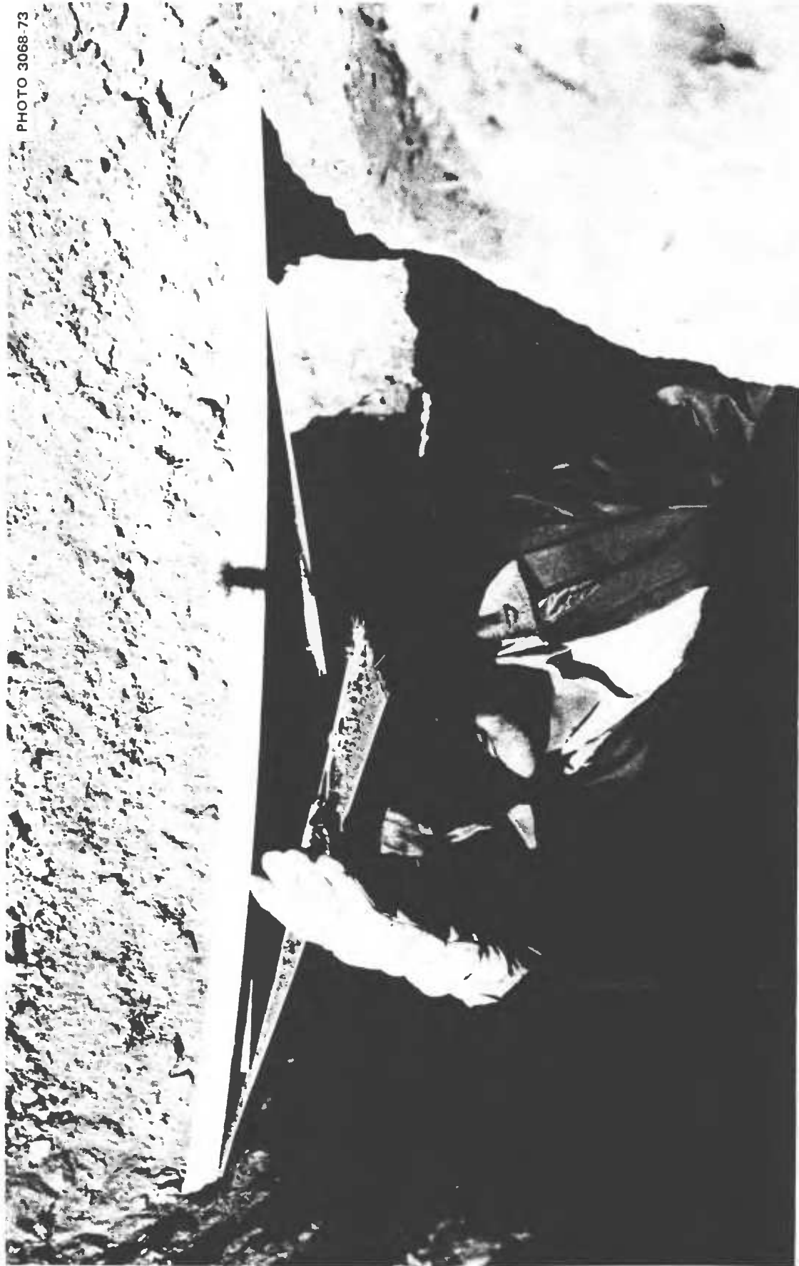
Fig. 3.9. View of the most damaged door after the removal of the adjacent door. Removal of some of the weight on the 1\frac{1}{2} X 1\frac{1}{2} -in. pine board that formed the unbroken frame of this door resulted in its becoming less bowed. The dry-earth bank pictured above this door appears to be vertical but actually was not. Kearny concluded that all that is needed to build a blast shelter in areas with stable and adequately deep earth is: (1) a deformable membrane (such as a tarp or rug) strong enough to support the weight of earth between it and the bottom of the earth arch formed by downward stresses and strains in the earth above the membrane; (2) the earth itself plus some practical although uncommon knowledge of how to use merely such a deformable membrane and earth to build a blast-protective roof over a trench.
